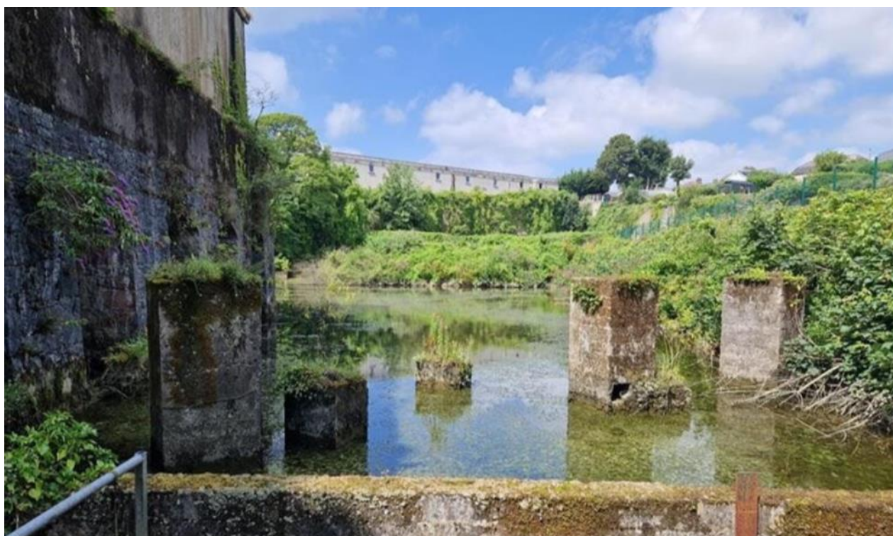
Figure 3-8 - View of Reservoir
