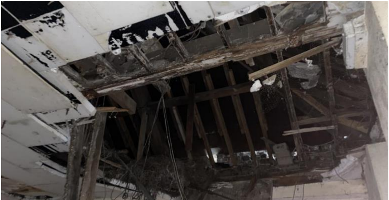
Figure 3-4 – Collapsing roof showing exposed timber structure within the Flaxmill building (photo taken from Phoenix ACM Survey report)
